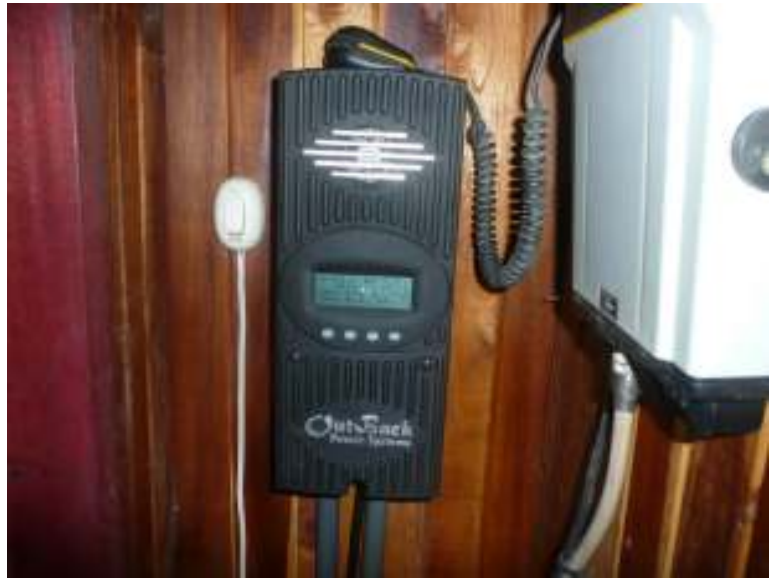
Charge controller and power “on-off” switch in power central closet.
